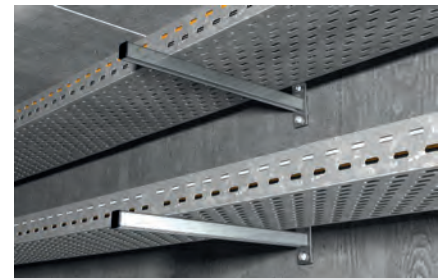
Cable tray on cantilever arm
