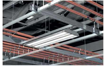
Supply lines on installation grid
