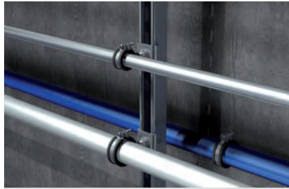
Lateral pipe mounting at channel
