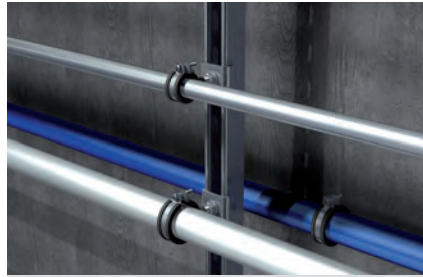
Lateral pipe mounting at channel
