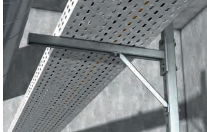
Cable tray on cantilever construction
