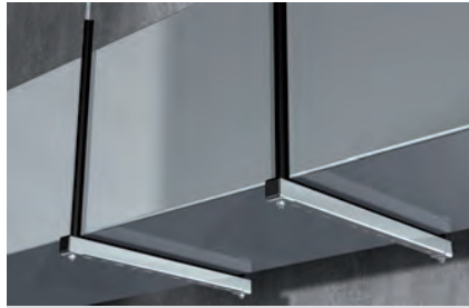
Air duct with sound insulation on installation channel
